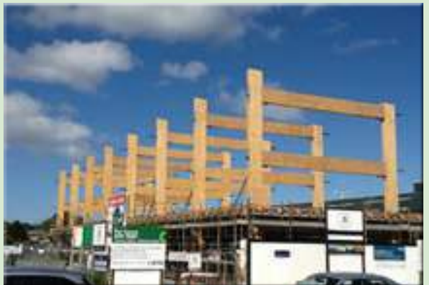
Young Hunter House, Christchurch. Timber chosen to minimise construction time and to facilitate a low damage design with high seismic performance.
