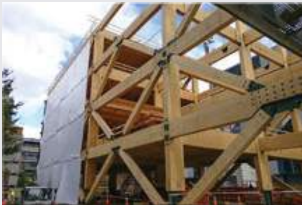
Beatrice Tinsley Building, Christchurch. Timber chosen to minimise weight of building, as existing foundations were reused. Also chosen to showcase PRES-Lam system pioneered at University of Canterbury.
