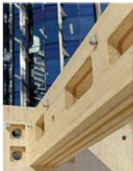
Penetrations in Beams for Services – International House Sydney. Lendlease Design. Photo: Ben Guthrie, The Guthrie Project.
