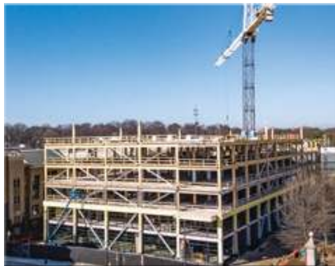
T3 Atlanta - 6 storey post and beam, over one story podium (StructureCraft Builders).
